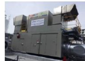
Hydrogen Gas Turbine (1MW class)
