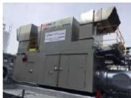
Hydrogen Gas Turbine (1MW class)
